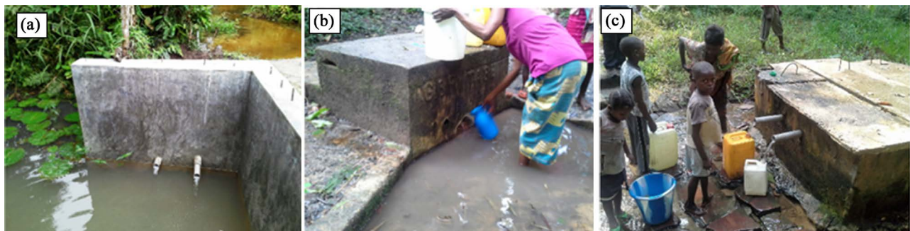
Figure 2. (a) and (b): Work without evacuation chanal creates stagnation; (c) Dilapidated work.
