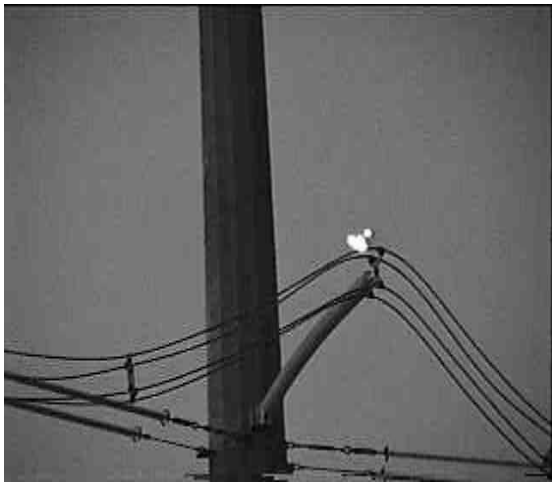
(a) Corona originating at the metal fittings of a 500 kV jumper line post NCI operating in a desert environment
