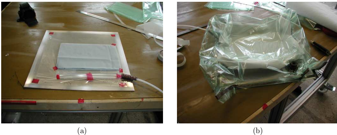
Figure 1.8: Scheme of the lay-up of self-manufactured parts; (a) The injection tube and fiber stack with peel ply can be observed; (b) The vacuum bag, the connector to vacuum tube, and the fiber stack with the breather material can be observed.
