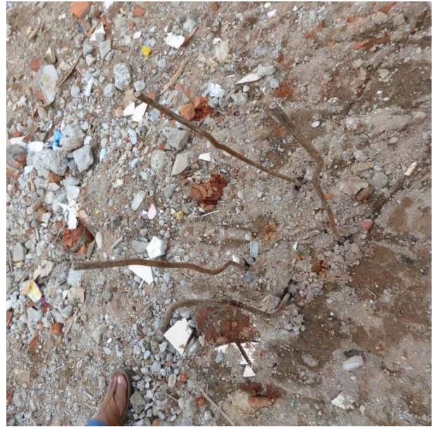
Figure 2. Heavily damage, use of column frame iron with a size that does not comply with regulatory standards
