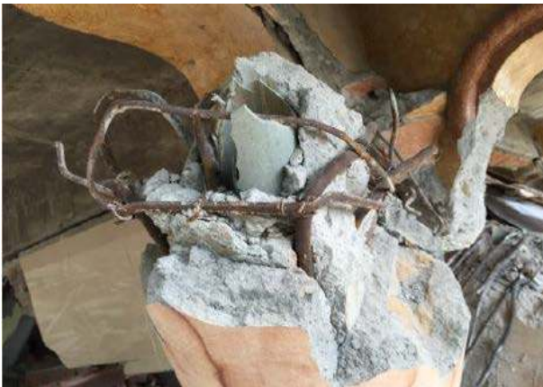
Figure 1. Moderately damage, planting pipes for the disposal of water located in the building column
