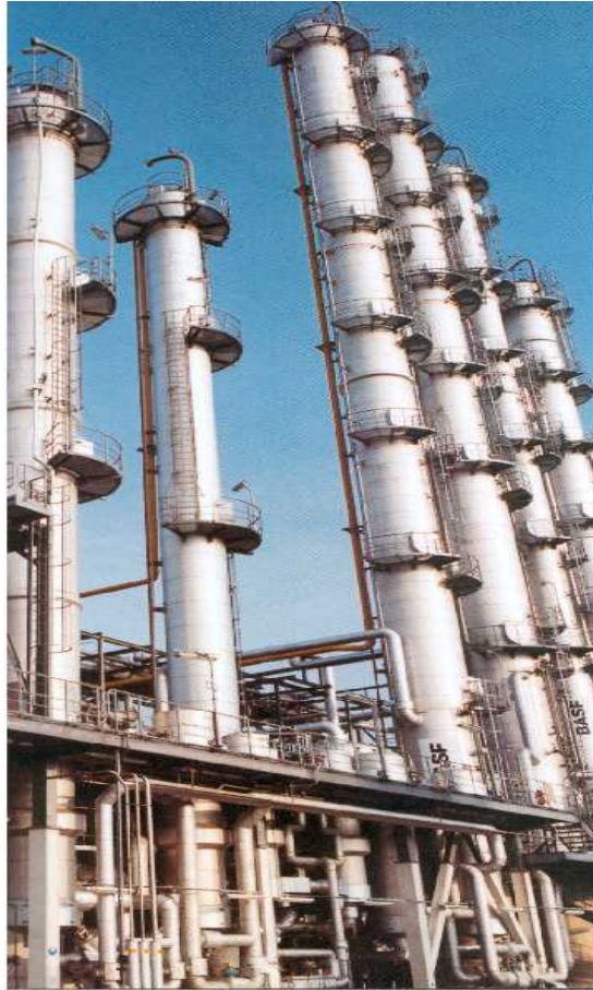
Fig. 12: Main packed columns for BASF NMP butadiene process /8/
