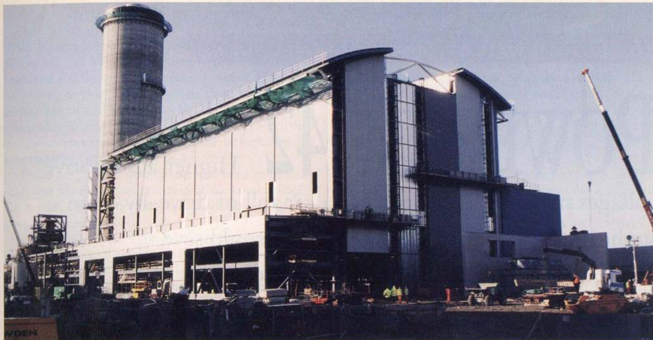
The turbine building at Baglan Bay will house the 9H gas turbine, its GE D10 steam turbine, and its NEM heat recovery steam generator.
