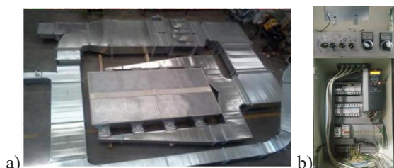
Figure 2. a) Ventilation system; b) Frequency converter
