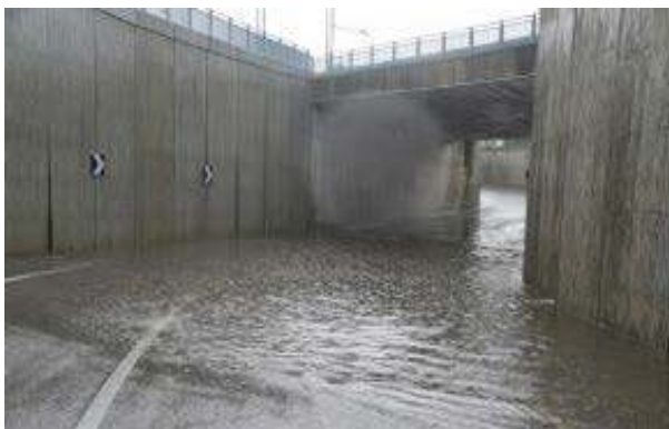
Figure 9. Underpass flooded in Pinerolo (Province of Turin, Italy). Courtesy from “L’Eco del Chisone” web journal ( www.ecodelchisone.it ).
