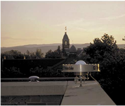
Fig. 12. Standardized GPS-choke ring antenna mounted on the roof of Lind Hall at Central Washington University. Similar installations are expected for universities interested only in atmospheric applications.
