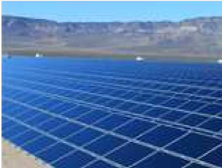
Figure 2 – 48 MW Copper Mountain solar electric power plant project in Nevada [71].
