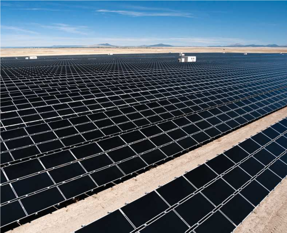
Figure 3 – 30 MW Cimarron solar electric power plant project in New Mexico [72].
