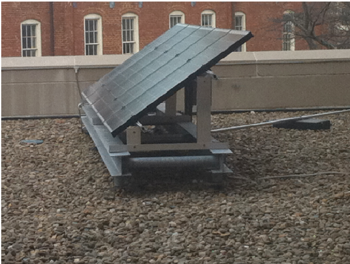
Figure 53 – Photovoltaic panels' setup.
