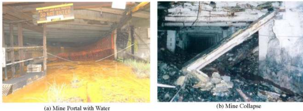
Figure 4. (a) “Yellow boy,” an iron oxide and sulfate deposit from acidic mine water. (b) An abandoned haulage-way. Abandoned for only a year, a roof beam collapsed bringing with it cabling, pipes, rock and roof bolts.
