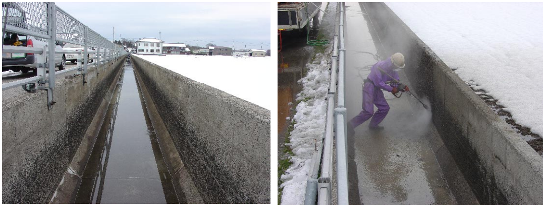
(a) Before repair
