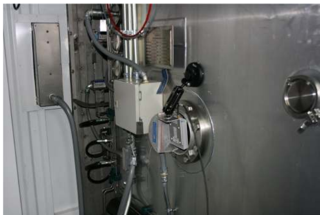
Fig. 9. Transmitter unit of a wireless system mounted at a site glass on a production-scale IMA Life freeze dryer by means of a suction cup
