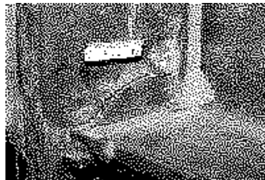
b. Column Flange "Divot" Fracture
