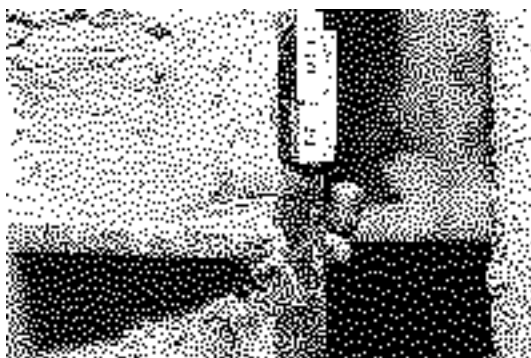
a. Fractures through Column Flange
