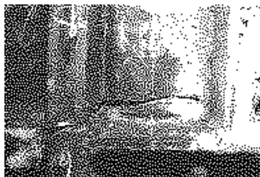
b. Fracture Progresses into Column Web
