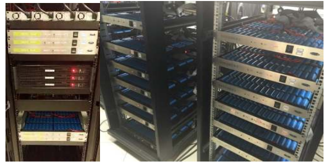
FIGURE 12. (a) Reconfigurable battery pack in UPS replacement in data centers; (b) The first large-scale reconfigurable battery system with 1792 LiFePO 4 26650 battery cells.
