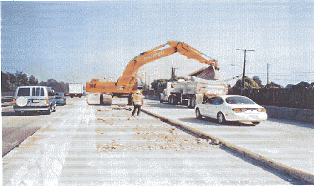
FIGURE 8 Precast concrete slab removal on I-10 pavement reconstruction project (photo courtesy of the University of California at Berkeley and the Innovative Pavement Research Foundation).
