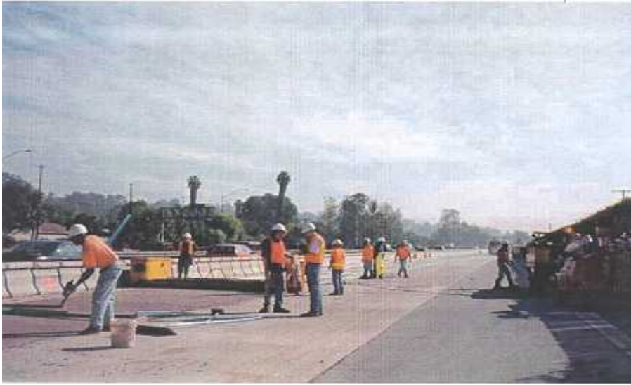
FIGURE 4 Movable barrier used to create a work zone on I-10 project in California.
