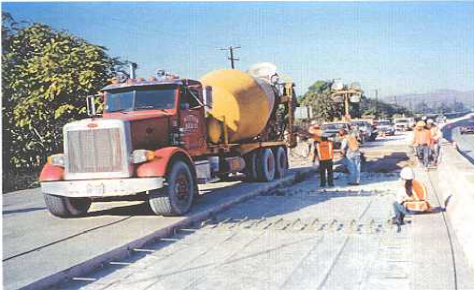
FIGURE 3 Placing fast setting concrete on I-10 freeway in California (photo courtesy of the University of California at Berkeley and the Innovative Pavement Research Foundation).
