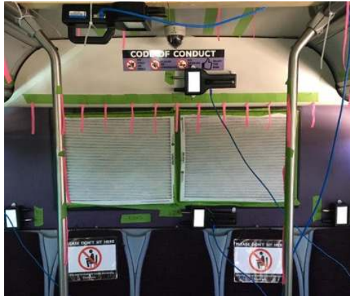
Figure S4: Application of 2 quantity MERV-13 air filters to the transit bus HVAC return air grille in the back of the bus.
