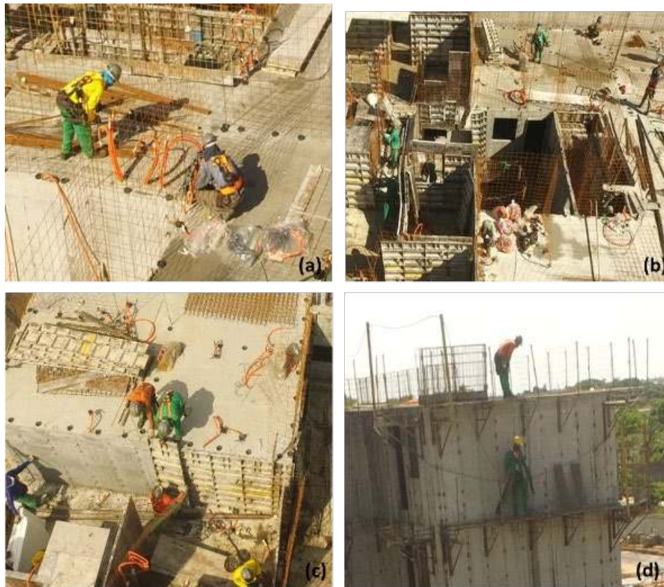
Figure 4 –Non-compliance identified in the concrete wall process
