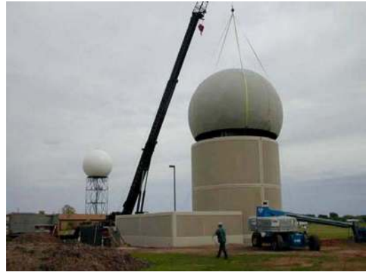
Fig. 1. Photograph of the NWRTPAR system during radome installation. The antenna array is housed inside the dome at approximately 12 m above the ground.
