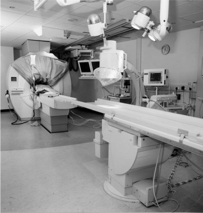
Fig. 1. XMR suite at Guy's Hospital, London, U.K. The change in the floor color indicates the transition from the MRI zone to the non-MRI zone.
