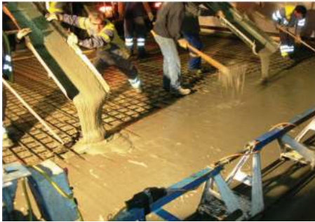
Figure 14. Cross section (dimensions in cm) with R-UHPFRC layer (in dark grey) and view of UHPFRC casting.
