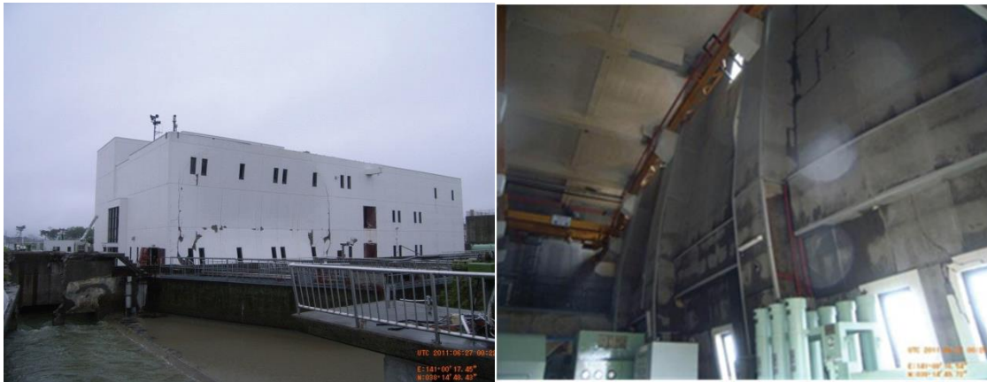
Figure 13 Minami Gamou Wastewater Treatment Plant out-of-plane flexure damage (a) exterior and (b) interior (Carden et al. 2012)
