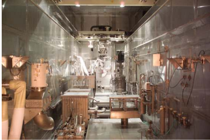
Figure 7. SNS target service bay (ORNL photo: 04118-2005).
