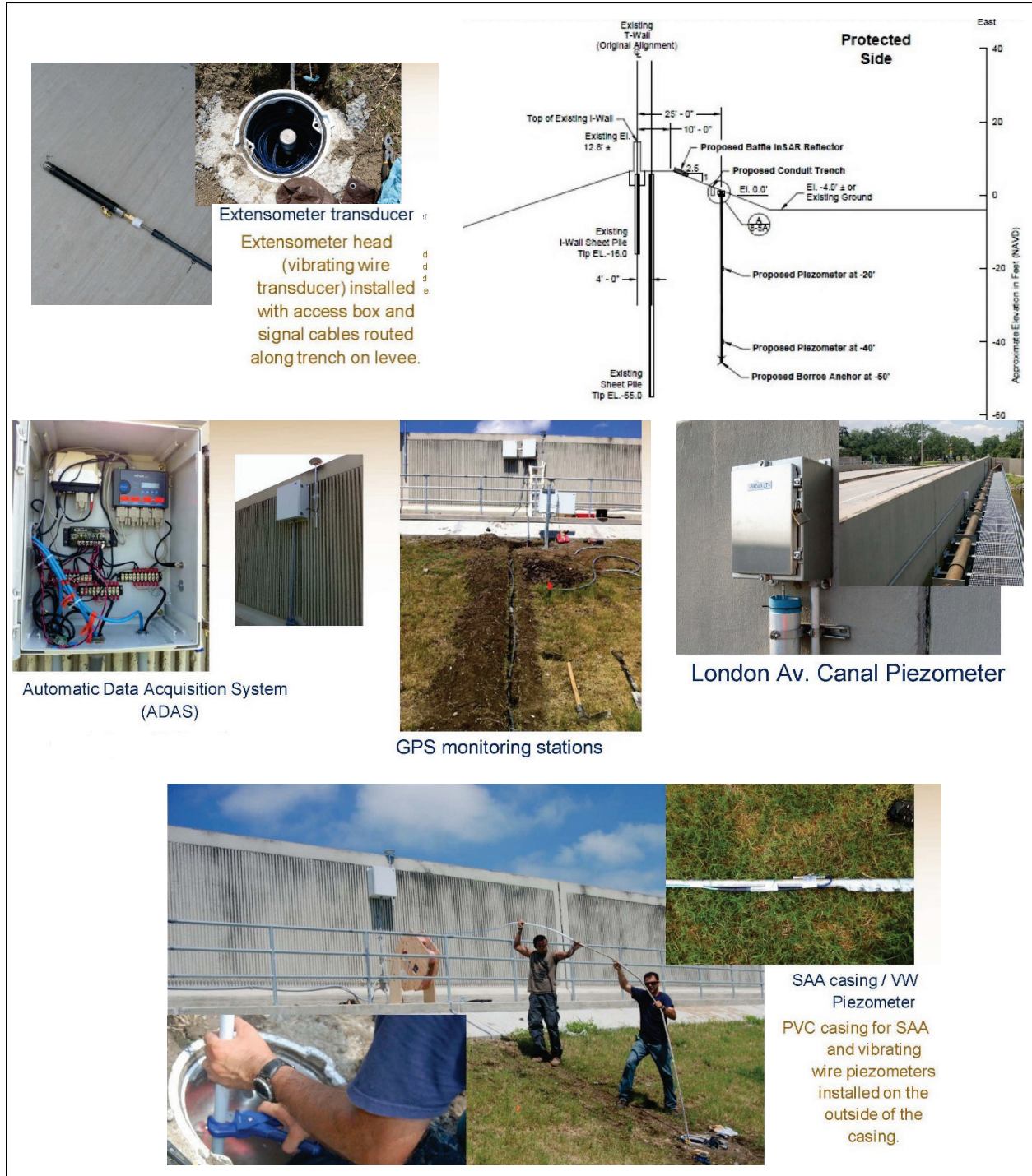
Figure 5-70. Monitoring at Site 8 at the site of the Hurricane Katrina Mirabeau levee breach on the London Avenue Canal. Monitoring technologies include piezometers in the canal and at levee toe, extensometers, GPS, InSAR reflector (see cross section), and ADAS system to log and transmit data (Brouillette 2012).
