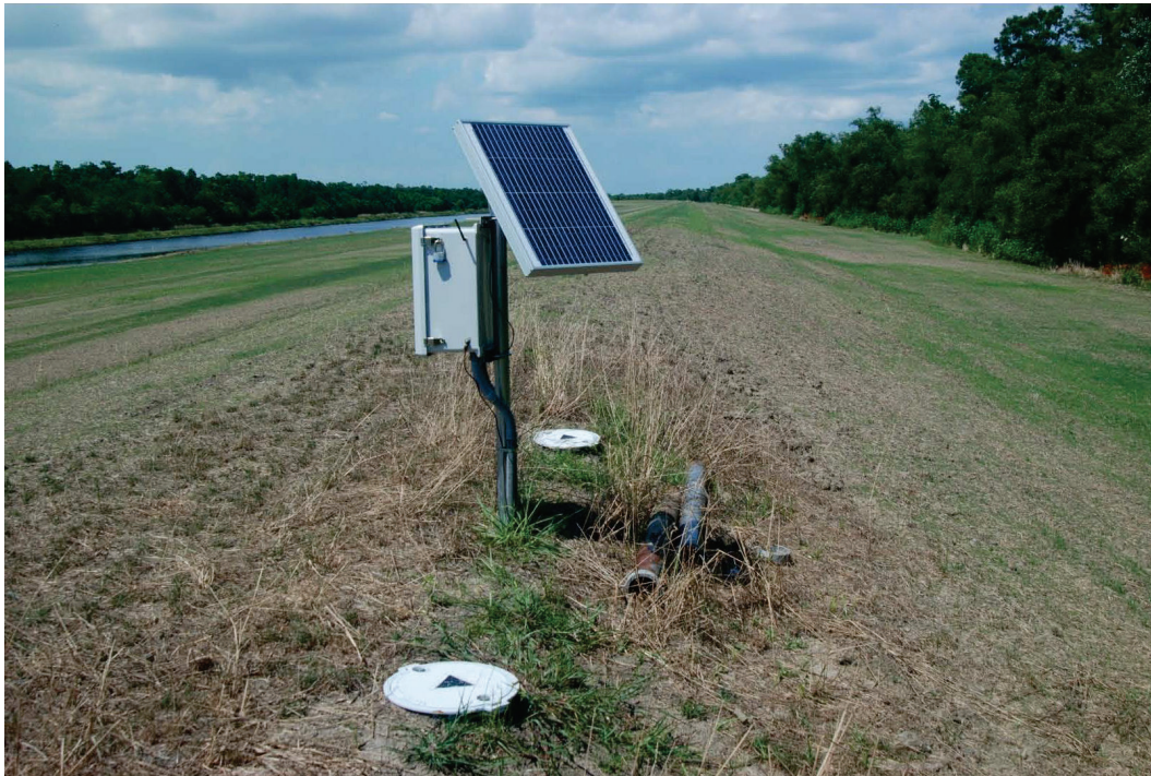
Figure 5-68. iLevee demonstration project at Site 2 on the V-line levee consisting of vibrating wire piezometers and in-place automated inclinometer (Brouillette 2012).
