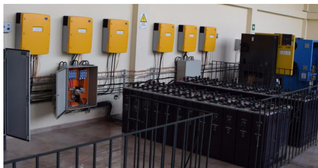
Figure 2. Installed battery bank and islanded inverters
