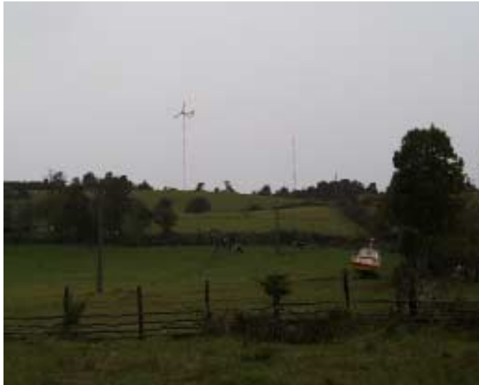
Figure 7. This Wind-Fossil Hybrid System Installed on the Island of Tac will Supply Full-Time Electricity to the 87 Families on the Island.
