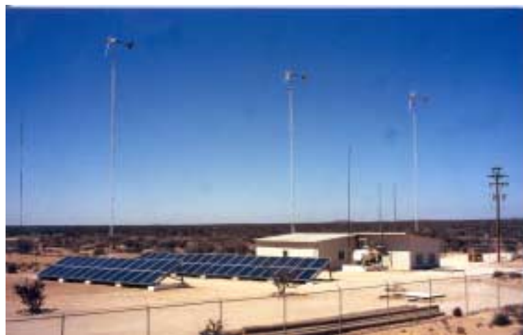
Figure 8. Wind-PV-Diesel-Hybrid Project at San Juanico
