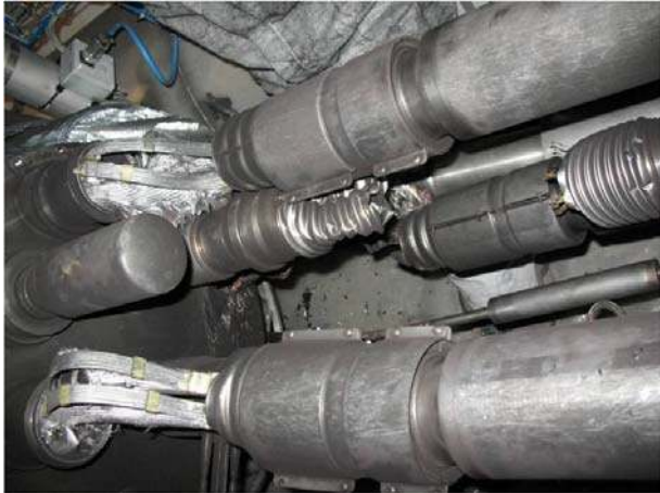
Figure 15: Damage to interconnection QBQI.27R3 by excess extension
