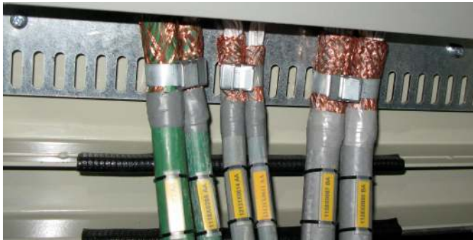
Figure 8.4: Stainless steel tie wraps.
