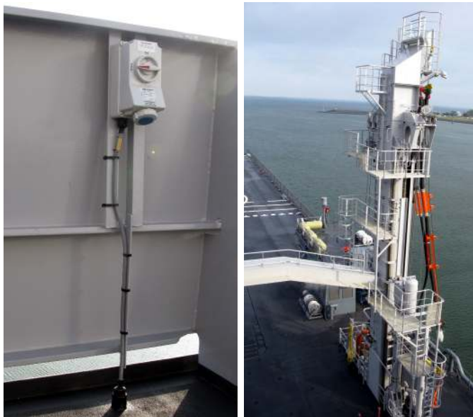
Figure 9.3: Power outlet and installation for Replenishment at Sea (RAS).
