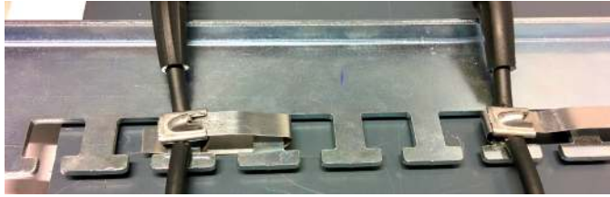
Figure 8.11: RG-58 and stainless steel tie wraps without a ground plane.
