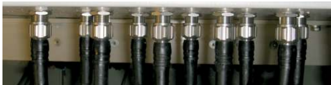
Figure 8.2: EMC cable glands at the entry of a shielded cabinet.
