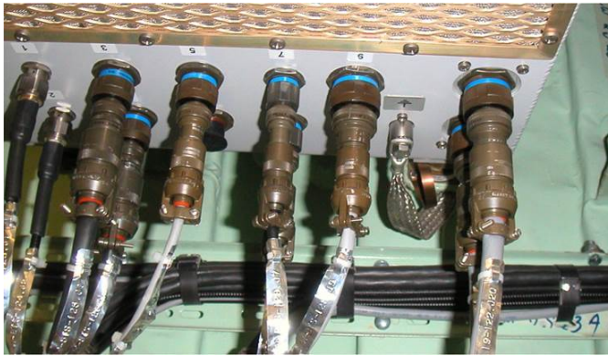
Figure 5.5: Connector plate as part of a shielding cabinet as an example of a current boundary type I.
