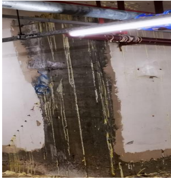
Figure 2. Cracking and water seepage of basement exterior wall
