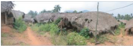
FIGURE 2: The rapidly ruined boat-shaped house of the Li nationality (investigated in Ocha Village, Dongfang City, Hainan Province).
