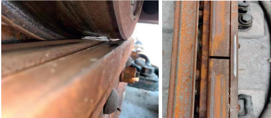
FIGURE 20: Impact on the top of the rail joint plate.
