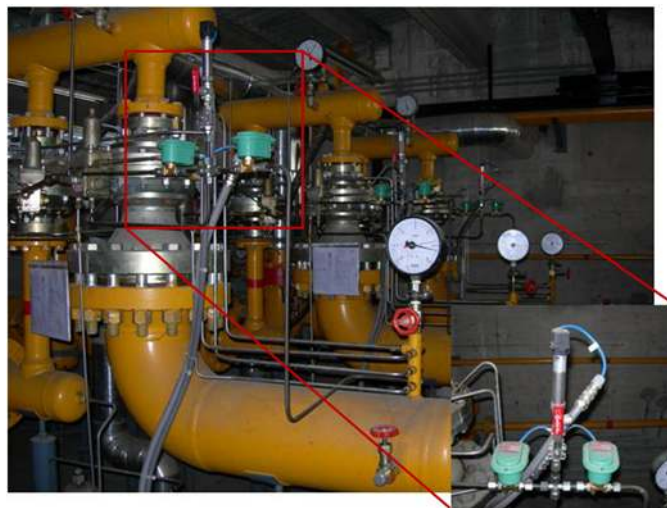
Fig. 15. Flow dividers installed in a M/R station
