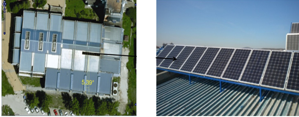
Figure 1: Installed PV system of 2 kW p in Niš.
