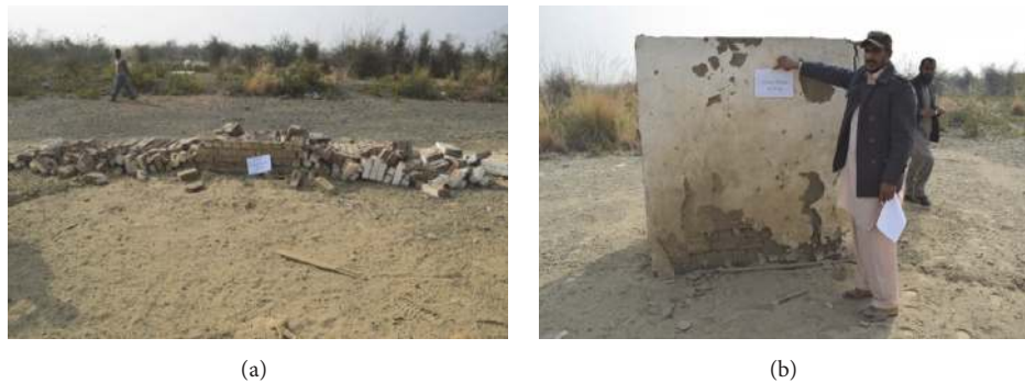
FIGURE 18: (a) Collapse of unreinforced masonry wall and (b) partially damaged but intact ferrocement wall.
