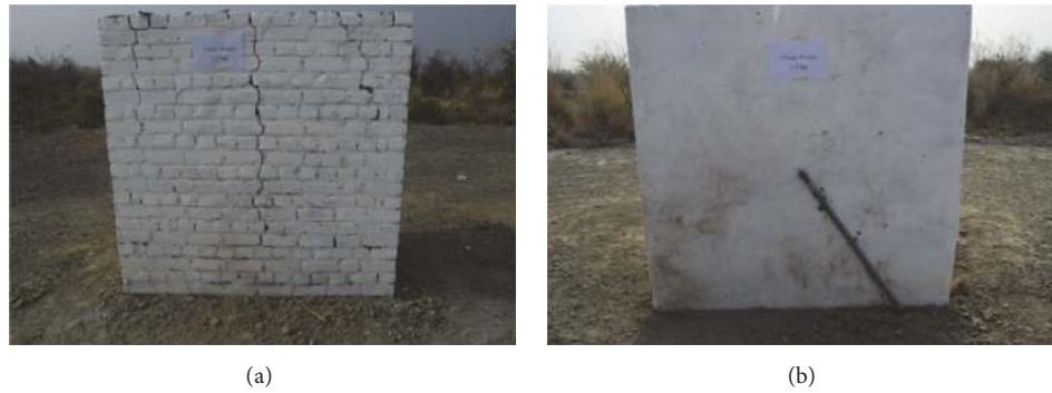
FIGURE 17: (a) Major shear and flexural cracks in unreinforced masonry wall and (b) no damage ferrocement wall.
