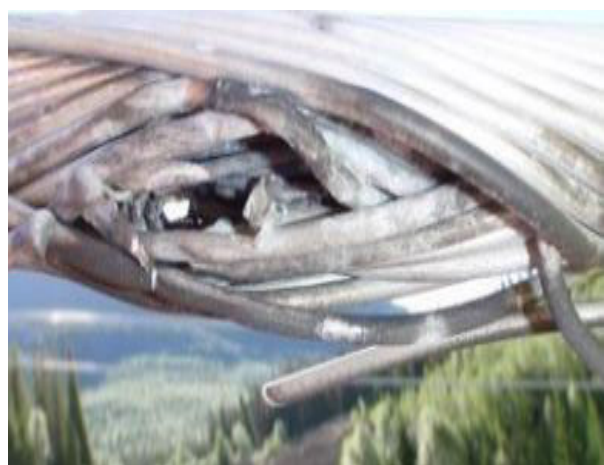
FIGURE 11. Lightning damage to conductor [105].
