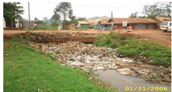
Figure Uganda_2: Blockage of drainage by plastic waste at Kyebando, Nsoba Zone (Kampala)
