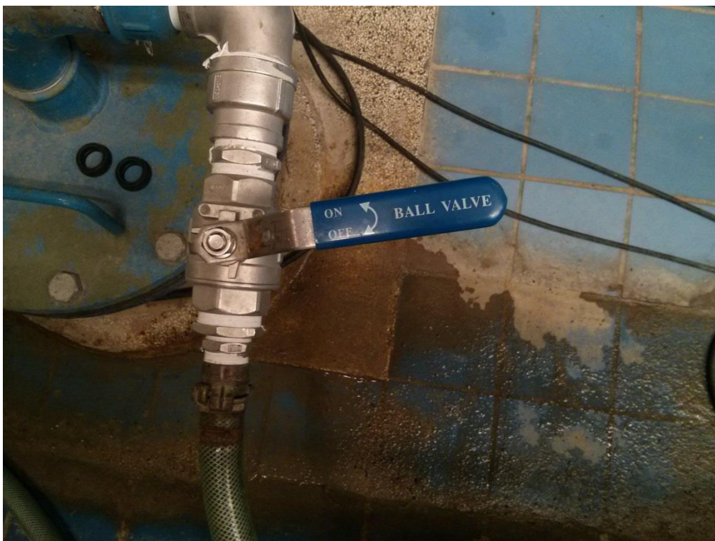
Figure H.8 – Ball valve to control water supply to flume
