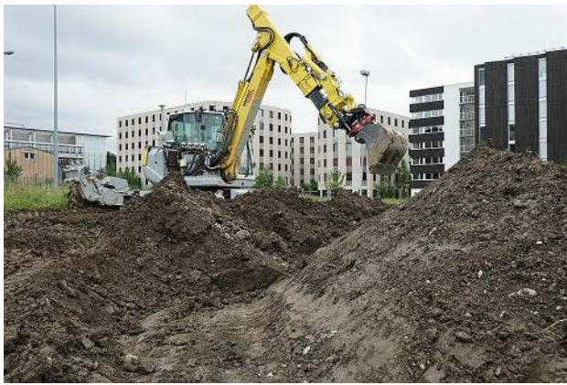
Fig. 1 The autonomous walking excavator HEAP can excavate free-form shapes with high accuracy. The image shows the s-curved embankment’s progress with the finished surface in the foreground and the unfinished pile to excavate behind it
