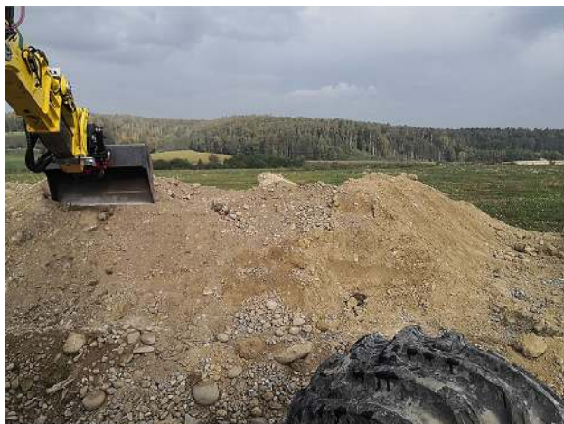
Fig. 19 The image shows the final state of the two-faced embankment experiment. An overall smooth surface finish with a clear and straight corner was achieved
