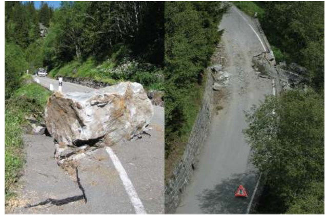
Fig. 1. Photography of a rockfalls event in 2006 that reached twice the road section near Le Plamproz, in the Bagnes Valley.
