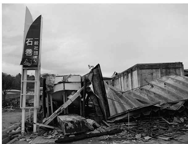
Fig. 4. IPA Hall after the Earthquake Photo by author.
