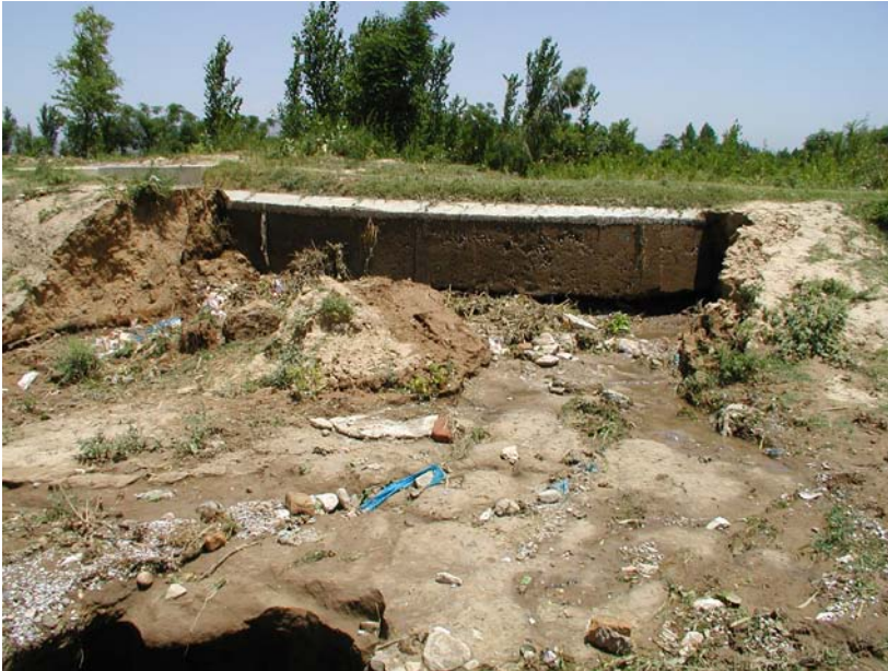
Figure 9.15.B. Berm erosion of a secondary canal due to overtopping
