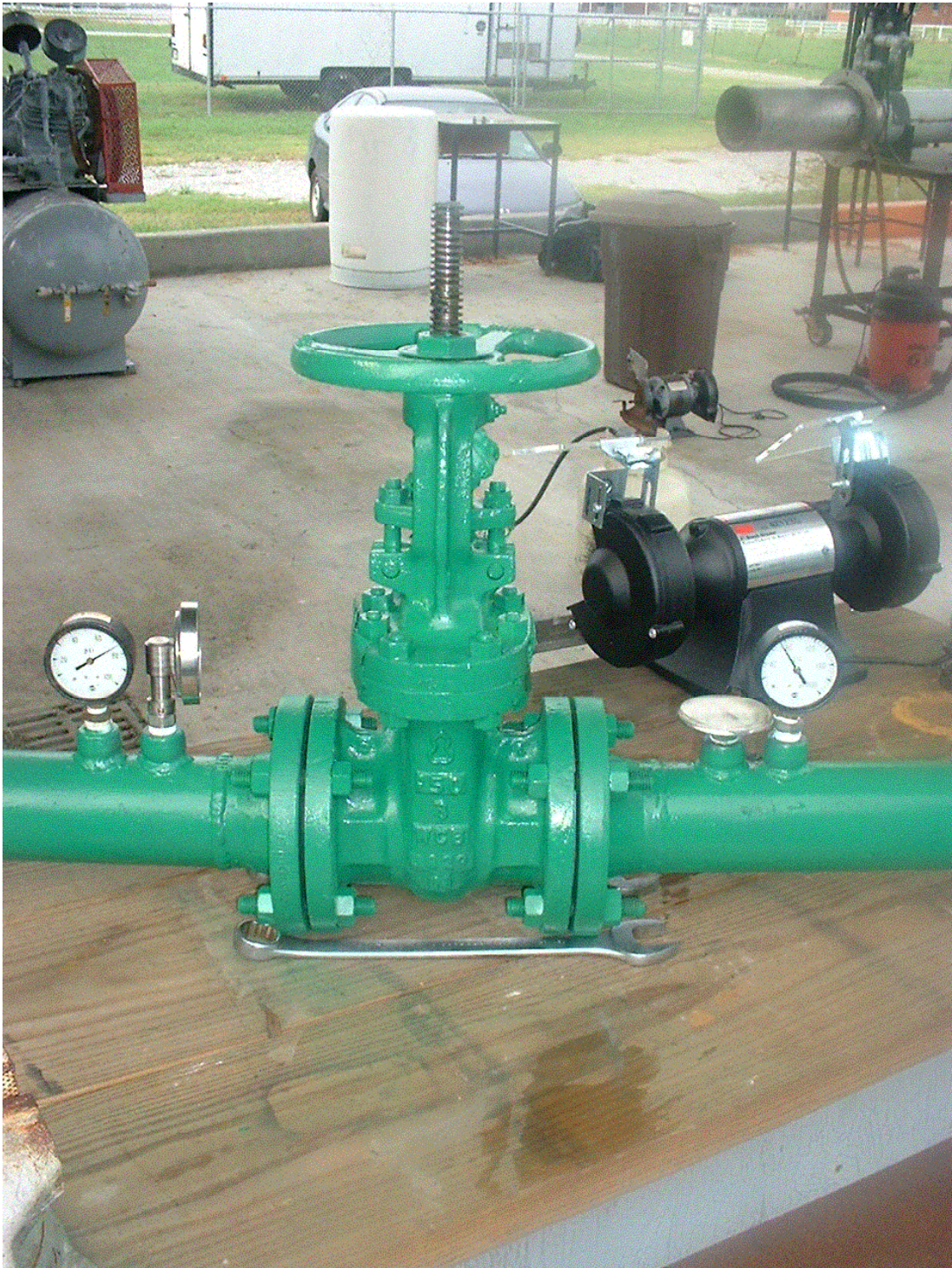
Figure 5.3 Fugitive Emissions Testing Apparatus
