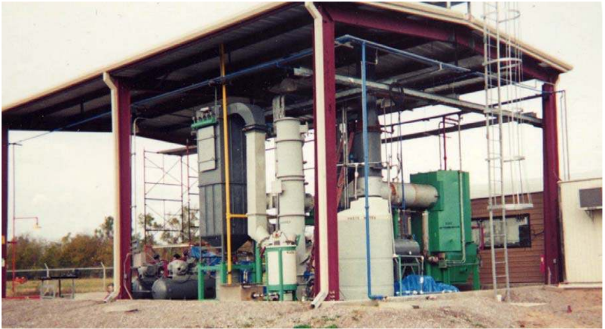
Baghouse, Scrubber, Wastewater Tank, and Afterburner
