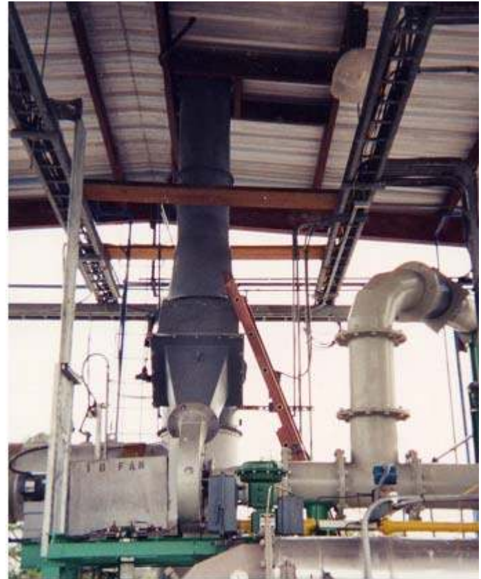
Induced Draft Fan and Stack
