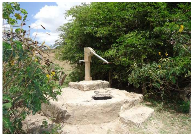
Figure 4. Unprotected and broken hand pump structure in Bubissa Kussaye community.
