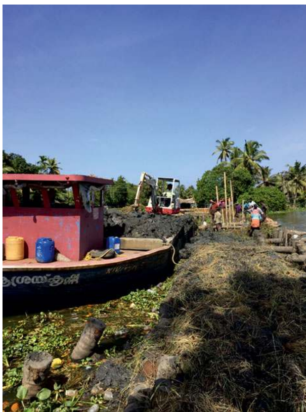
Figure 5. View of the bund reconstruction efforts that secures Kanakassery, Valiyakari, and Meenapally paddy polders from the Vembanad Lake in Kuttanad. The left of the bund is the Vembanad Lake and the right of the bund is the paddy polders that span over 750 acres.
