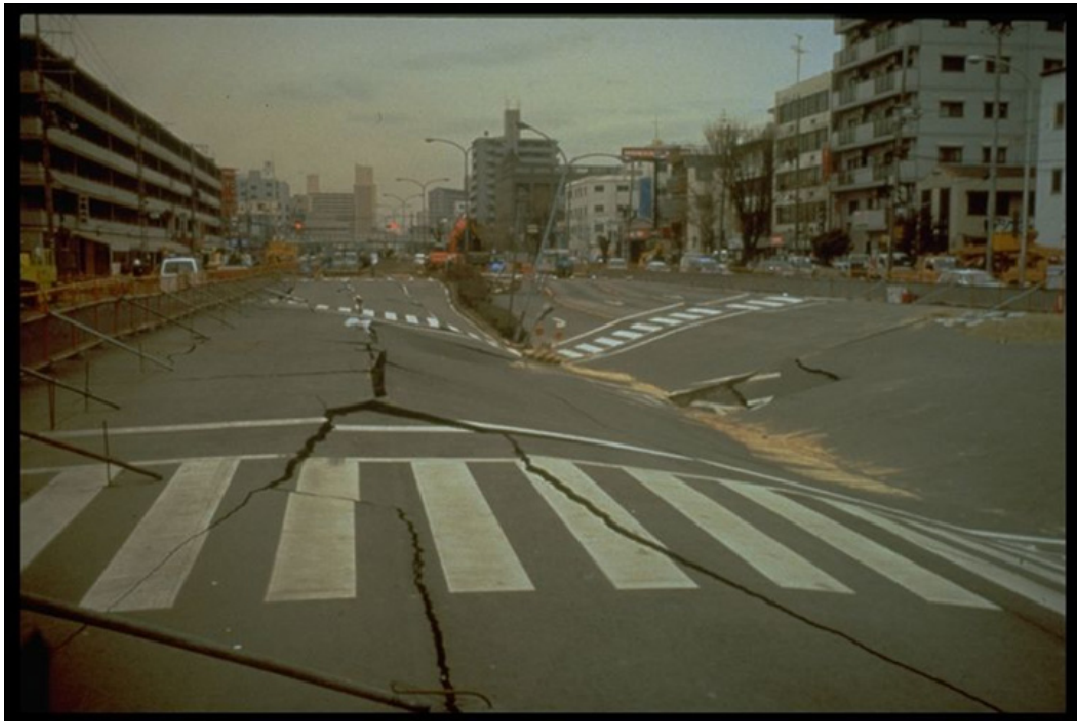
Figure 2.6 - Ground subsidence on road above the Daikai station (from Sitar 1995)
