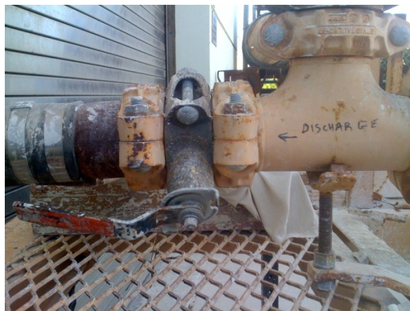
Figure A.7 - Valve set to DISCHARGE (one of two valves)
