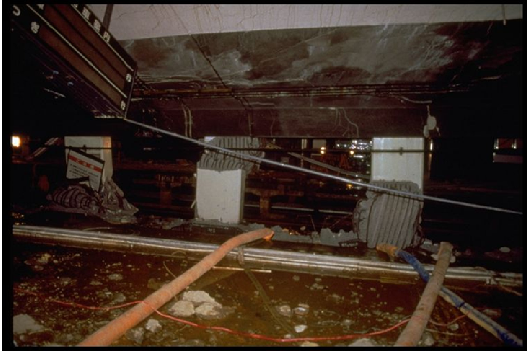
Figure 2.5 Damage to unconfined interior columns, leading to roof slab collapse in the Daikai subway station (from Sitar 1995)
