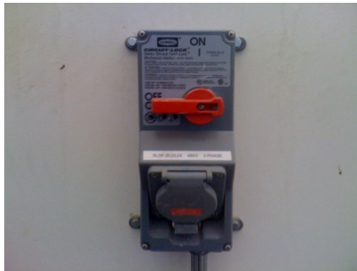
Figure A.2 - 460V power outlet
