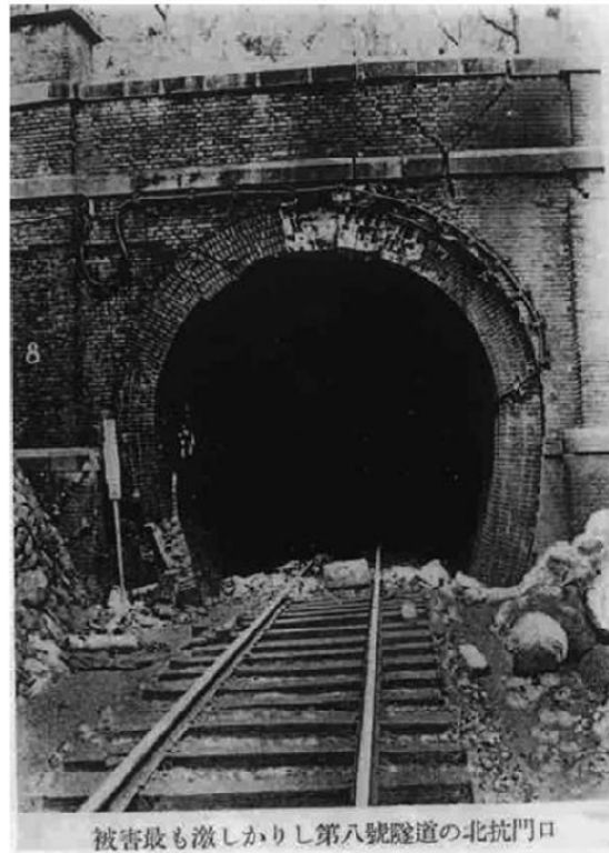
Figure 2.10 Damage to the old Sanyi No. 8 south portal after the 1935 Hsinchu-Taichung earthquake (from Hwang and Lu 2007)
