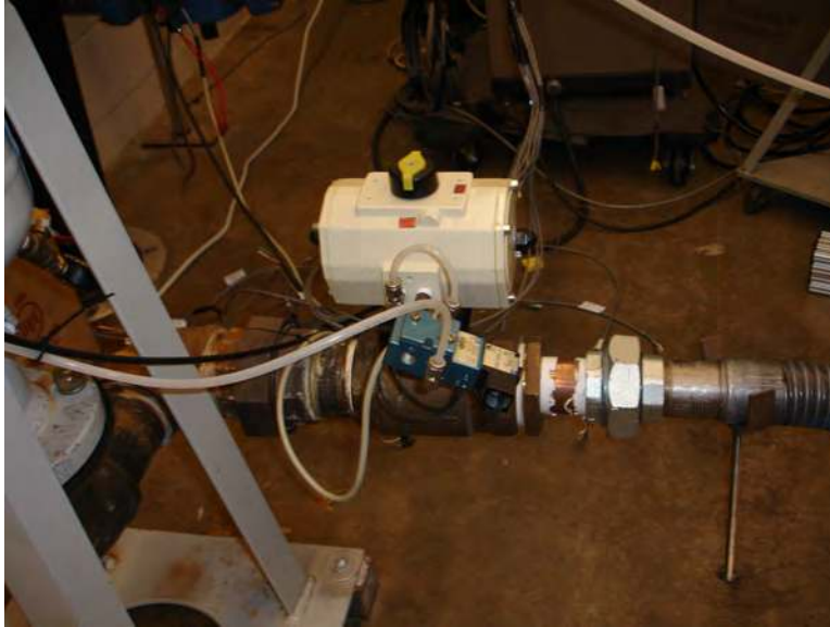
Figure F.8: High pressure ball valve and controller
