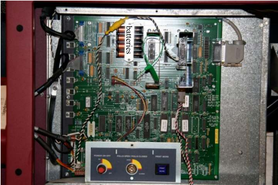
Fig. 3. Circuit-board cover removed from motherboard enclosure. Bottom center, panel for on/off knob. Top center (just to the right of “batteries”), a green strap seal remaining after the circuit-board cover has been moved past it (see discussion of seal regime #1). Slightly to the lower right of center, 1 configuration ROM and 3 program ROMs with white labels. At top left and top center of enclosure, one can see two of the 10 threaded holes for the screws that hold the circuit-board cover in place.
