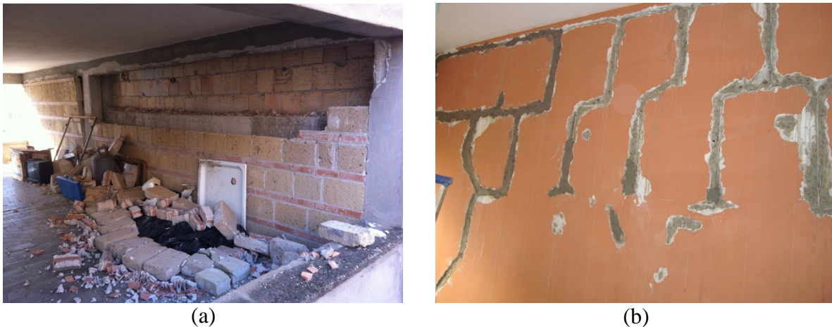
Figure 1. Damage to (a) infill walls and to (b) internal partition after a 4.9 M_w Italian earthquake.
