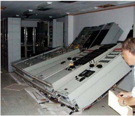
(a) Seismic damage to anchored cabinets in 1985 Mexico Earthquake (Magnitude 8), FEMA 74 (2011),
