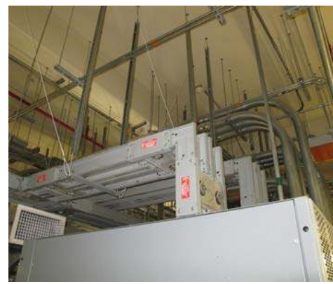
(b) Electrical Busway Enclosure
