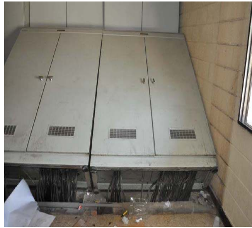
(b) Seismic damage to unanchored cabinets in 2010 Haiti Earthquake (Magnitude 7), FEMA 74 (2011).
