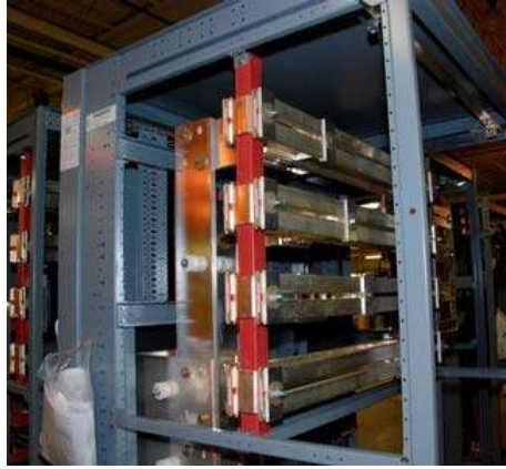
(a) Copper busbars
