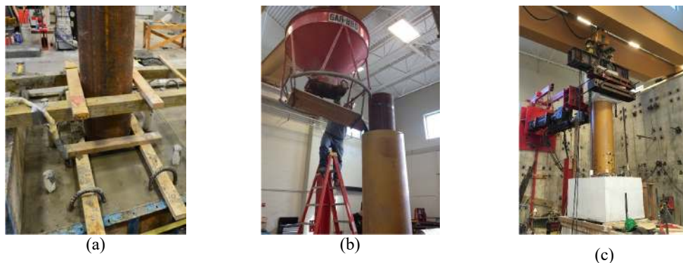
Fig. 2. Constructing procedure (a) footing casting around the inner steel tube; (b) placing the FRP tube and pouring the concrete wall; (c) the HC-FCS column
